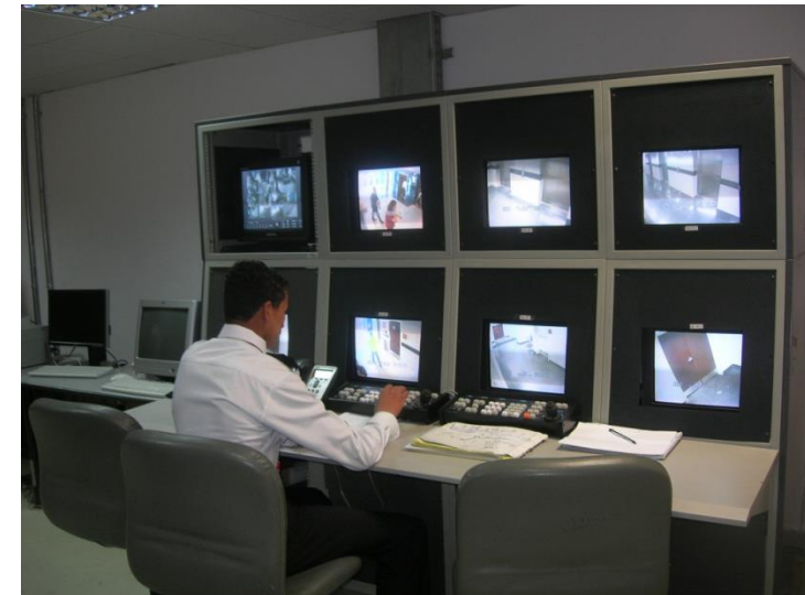
FCC MONITORING FACILITY
